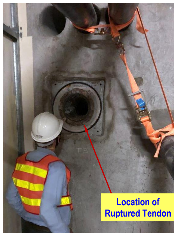
Figure 9 Photo at Pier P5 with Location of Ruptured Tendon T3
