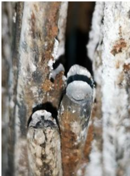
Figure 14 Broken corroded wires with cup-and-cone failure feature
