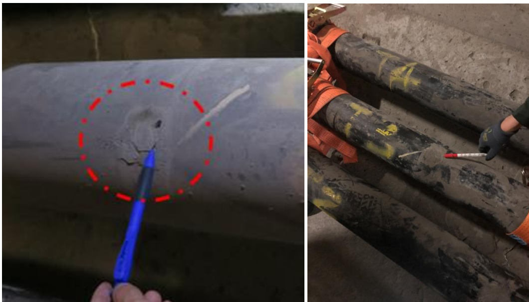
Figure 24 (Left) Grout Injection Point observed on ruptured Tendon T3; (Right) Trace of grout injection points of tendons on symmetrical parallel side
