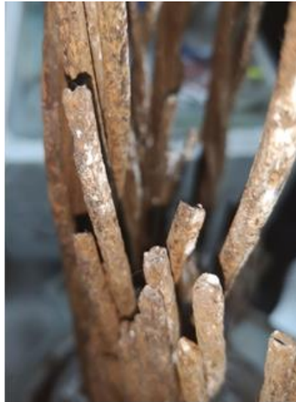
Figure 12 Broken strands with significant reduction in cross section
