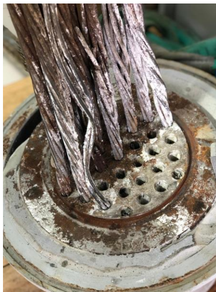
Figure 13 Ruptured wires pulled out from anchor head
