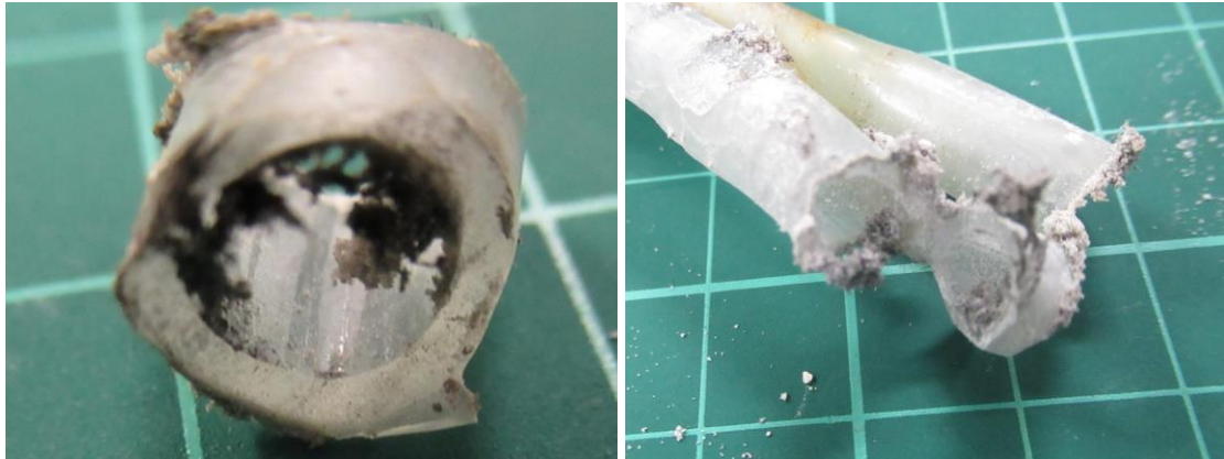
Figure 20 Trace of residue within air release tube at anchor head P5
