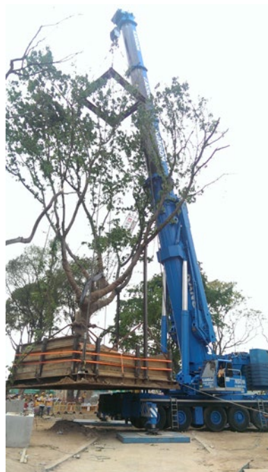
Mobile crane with lifting capacity of 500 ton is used for tree transplanting. Steel container is fabricated to house the root ball for transplant.
