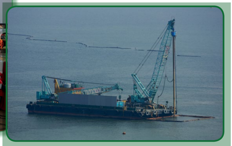
Water Pollution Abatement - Perimeter Silt Curtain Enclosing the Site and Localized Silt Curtain for Major Construction Works
