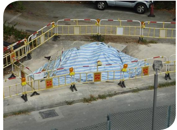
Cover Stockpiled Construction and Demolition Materials with Impervious Sheet
