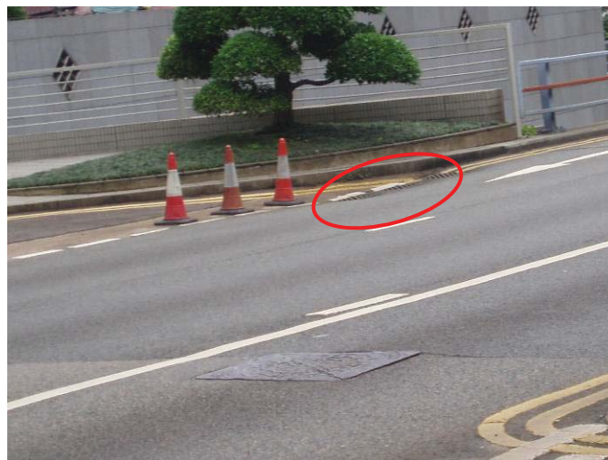
Multiple gullies near junction
