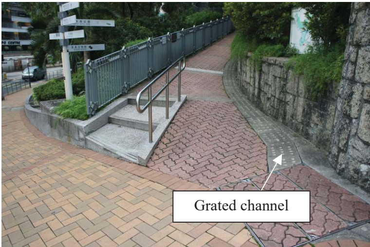
Interception channel at entrance/exit
