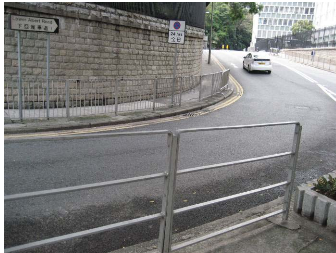
Multiple gullies at sag point/junction
