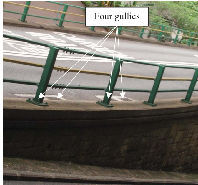
Multiple gullies at sag point
