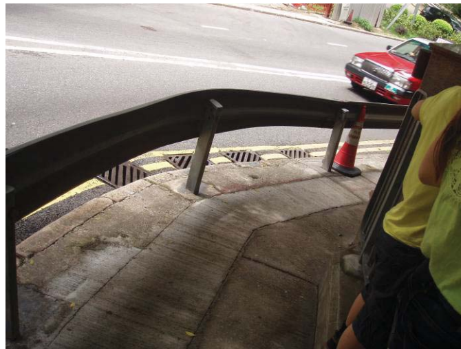
Multiple gullies at kerb opposite to the junction
