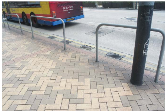
Multiple gullies near junction
