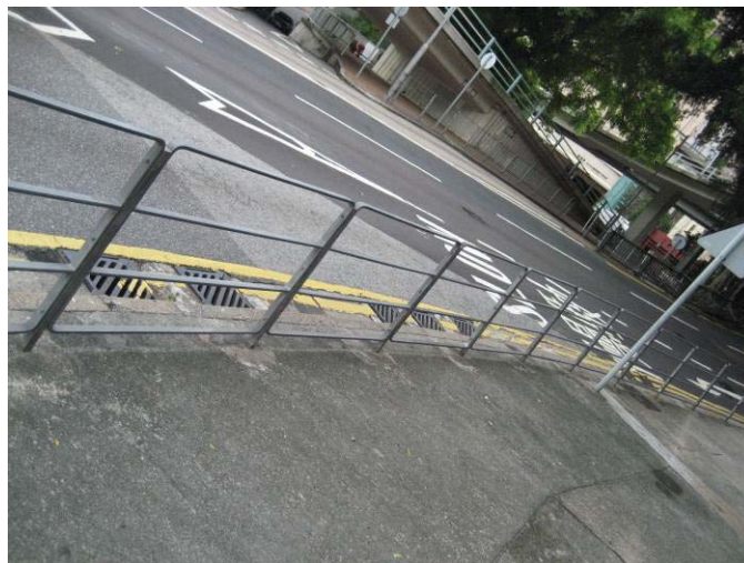
Multiple gullies at sag point/junction
