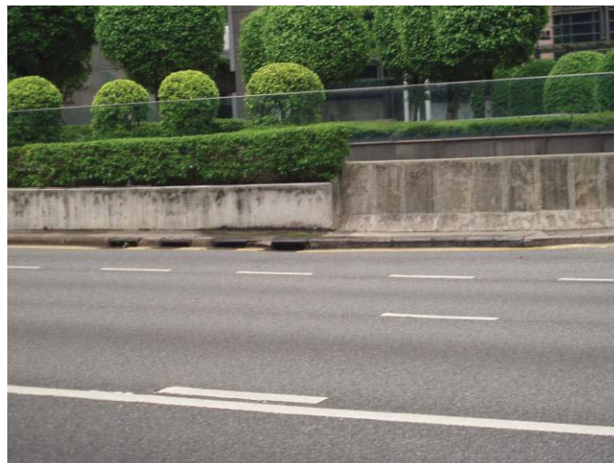
Multiple gullies near junction
