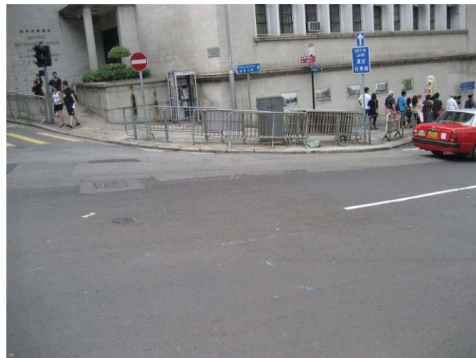
No gully near the junction
