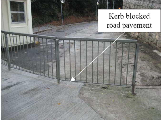
Kerb blocked road pavement
