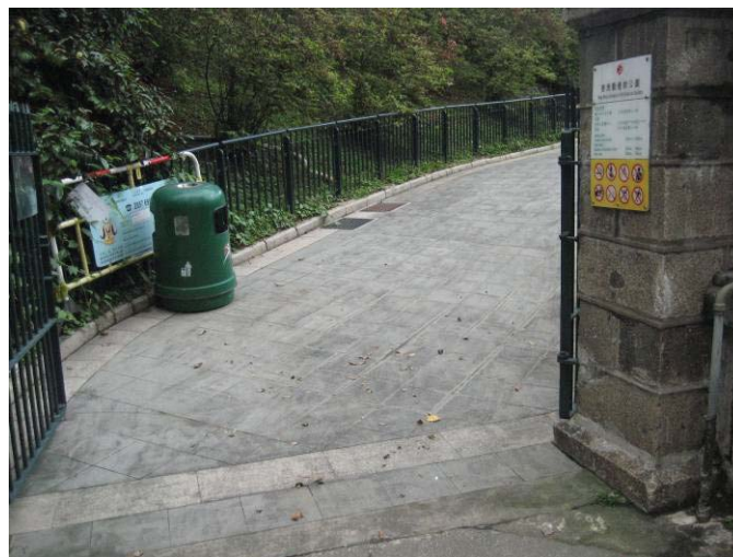
No interception channel at entrance/exit
