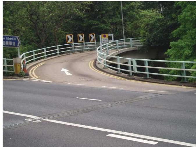
No gully near the junction
