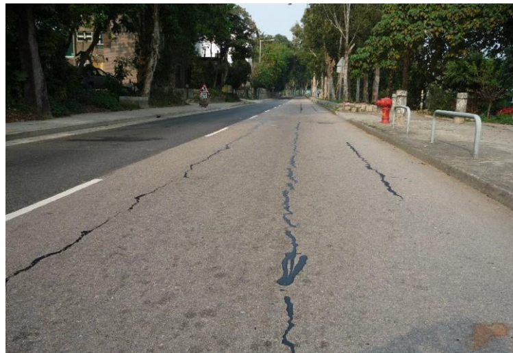
Photo 1 – Filling of wide single longitudinal cracks caused by the adjacent trench excavations
