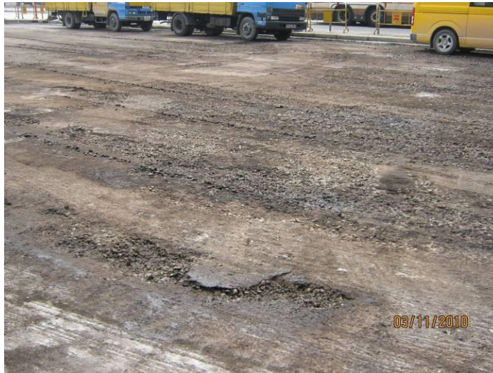
Photo 3 – Disintegrated base layer materials exposed after cold milling
