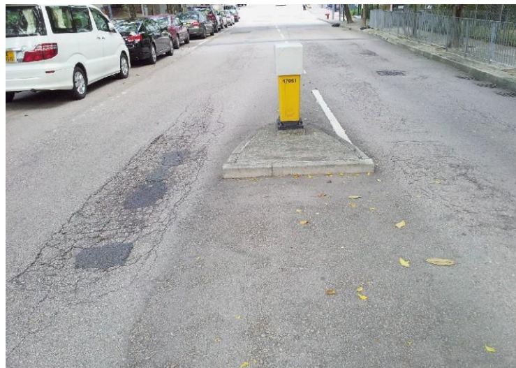
Photo 5 – Severe surface distress requiring deep inlay
