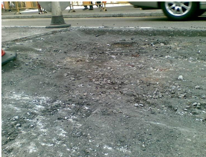
Photo 4 – Disintegrated base layer materials exposed after cold milling
