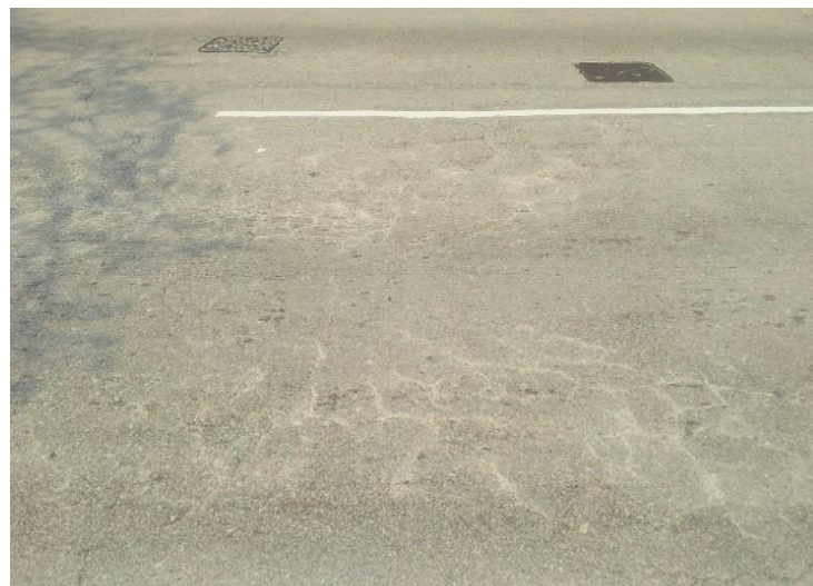
Photo 6 – Sign of pumping from lean concrete base
